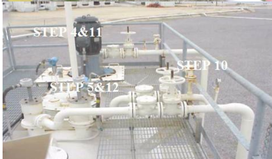
Cleaning OWS – OWS Sump
