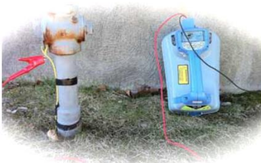
Direct connection to gas service tracer wire
