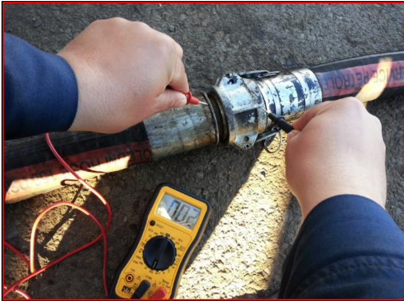
Shown here, testing a hose to hose bond connection using a Multimeter
